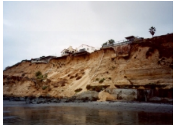
Upper bluff failure in Encinitas. Note sea wall at lower right.
