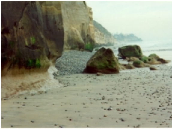
Sand and cobble beach. Note beginnings of notch and large sandstone blocks from previous bluff failure.
