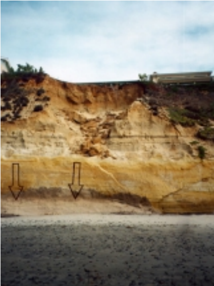
Notch fill. Note colored material used to blend with natural bluff face.
