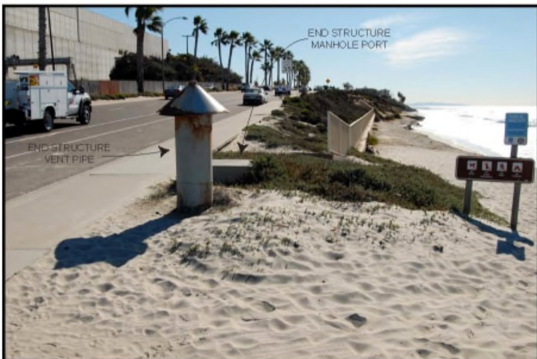
Photograph of end structure taken January 2013. The round vent and manhole access port of the underpass end structure are all that is visible of above the beach sand. Approximately 10' of the end structure's 16'-7-1/4" length is located underneath Carlsbad Blvd. and the sidewalk shown in this photograph.
