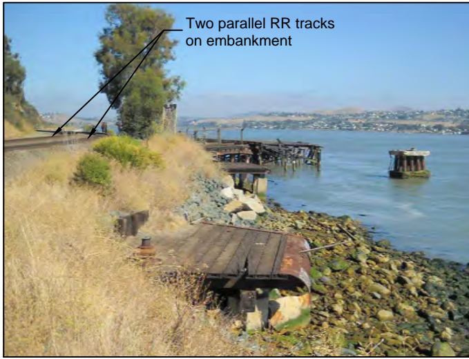
Photograph of existing structure to be deconstructed as shown in sections A, B, C, D, and E
