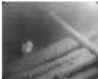
Steam and water piping connecting boilers and pistons.
